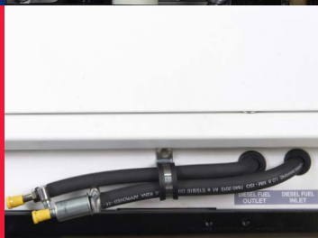
Input/Output fuel pipe
