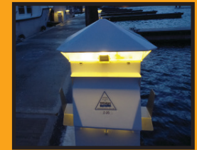
Protected kWh Counter
