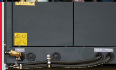
Input/Output fuel pipe
