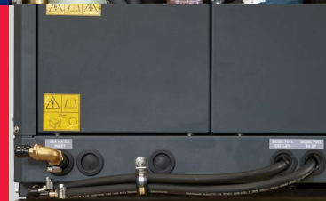
Input/Output fuel pipe
